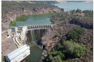
The Copco No. 1 dam on the Klamath River is slated for demolition in 2024. Photo by Stormy Staats/Klamath Salmon Media Collaborative
