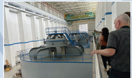
Northern California Tour participants view the giant turbines inside the Shasta Powerplant, just below Shasta Dam.
